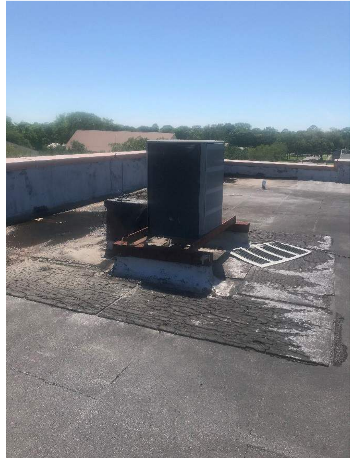
MECHANICAL UNIT ON HOUSE ROOF
