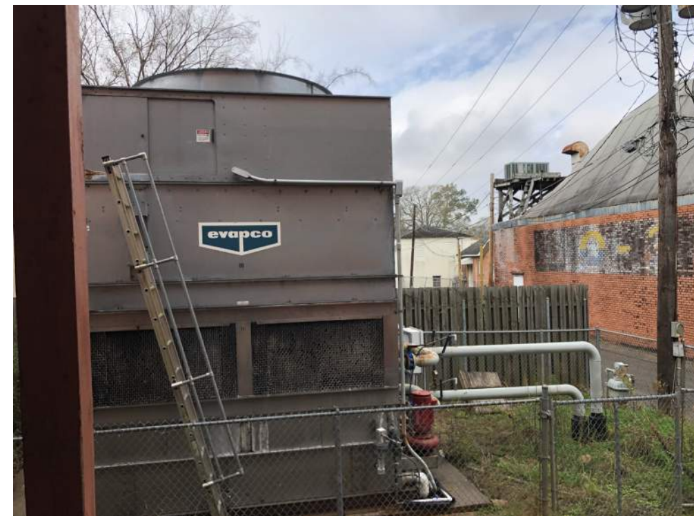
EXHIBIT A - COOLING TOWER
