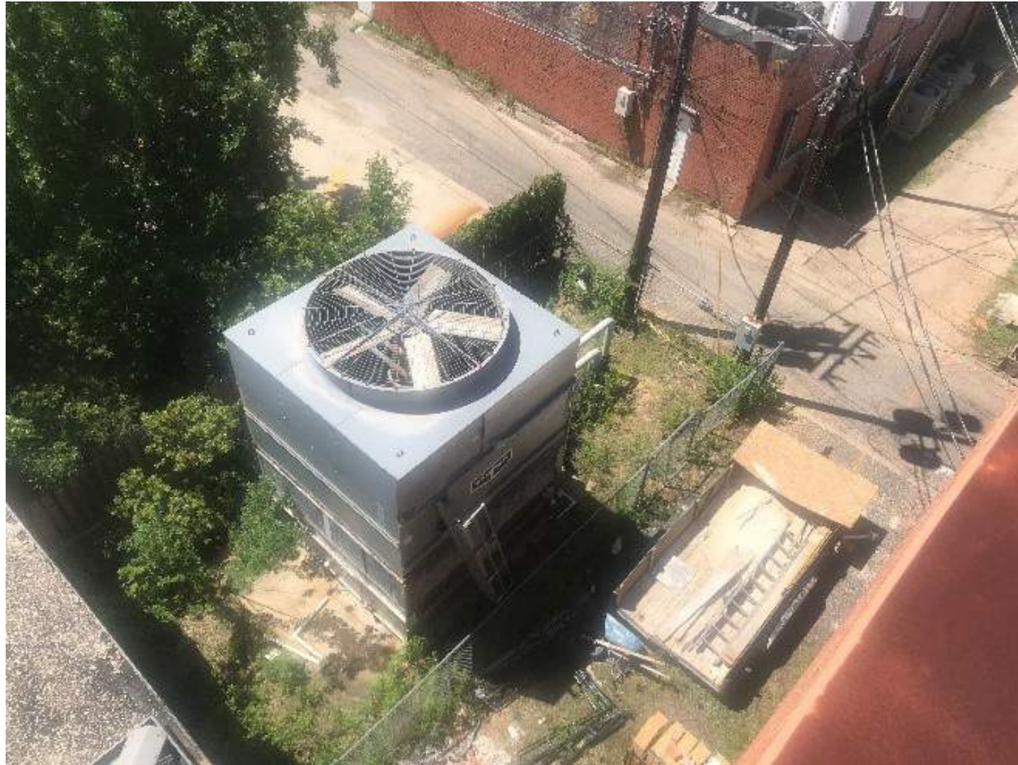
LOOKING DOWN ON MECHANICAL YARD
